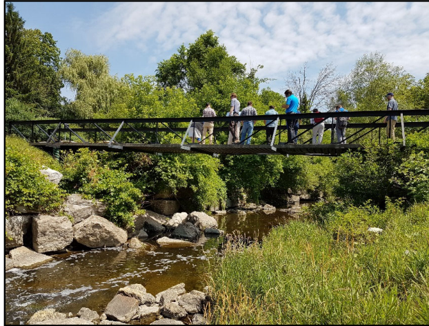
Condition: Needs Repair
