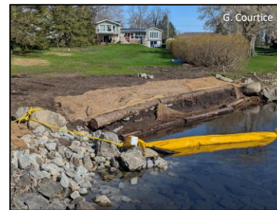
Failure caused by challenging construction conditions
