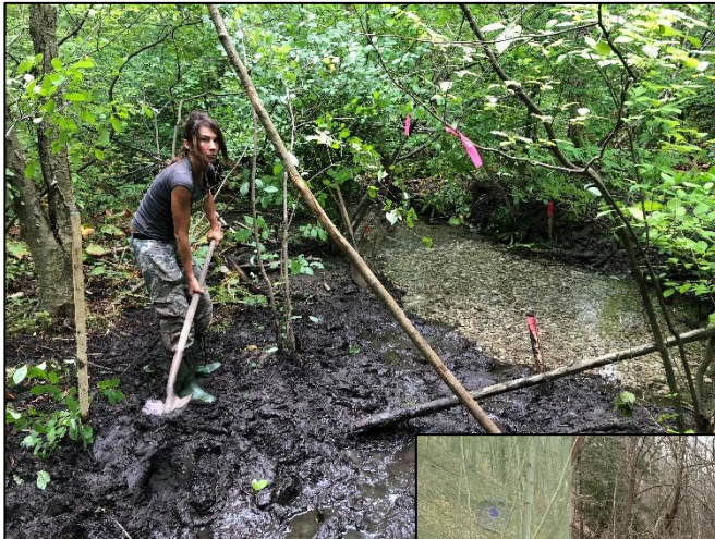
Finger drain and gravel pad, NPCA, upper 12 Mile Creek, 2018 Source: I.D. Smith
