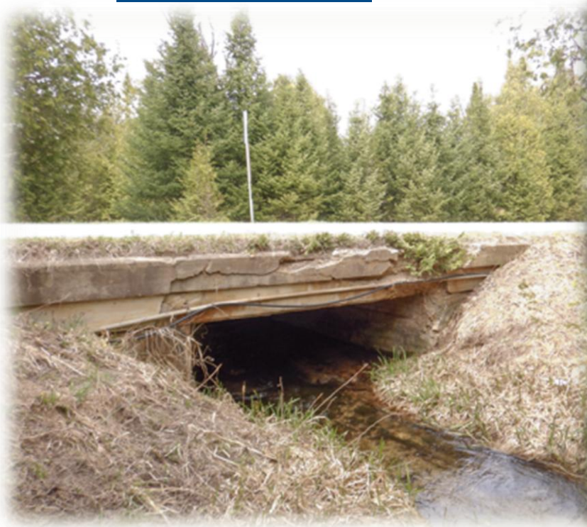
Degraded “cast in place” open foot culvert
